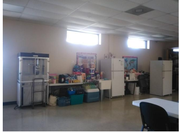
Everything had to be removed from the concession stand for the renovations.
