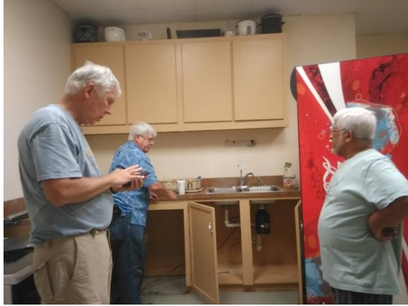
Lions Chuck, Bob, and Mazher continue to dismantle the kitchen prior to painting.
