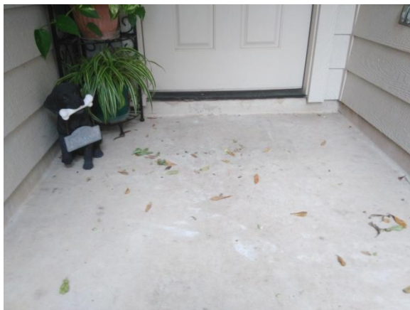
The front door with 5 inch drop to concrete before ramp.
